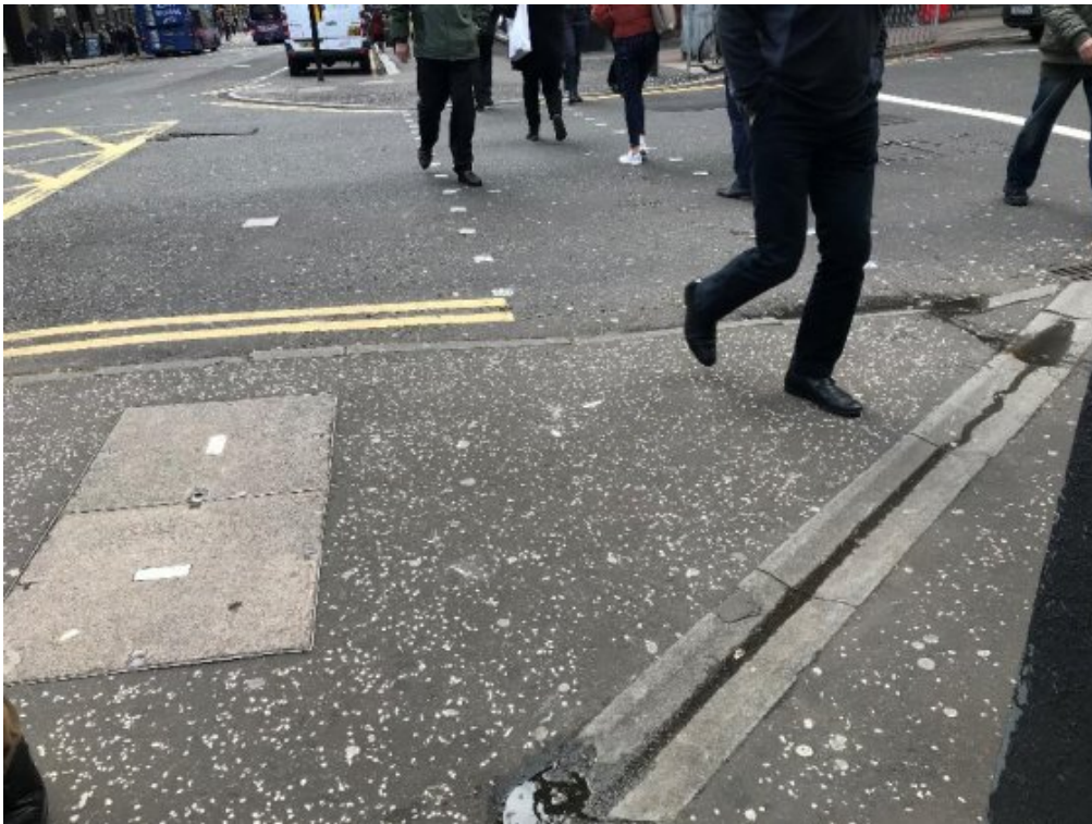
Figure 8: Tactile paving absent from signalled crossing, despite recent maintenance resurfacing. Channel drain issue.
