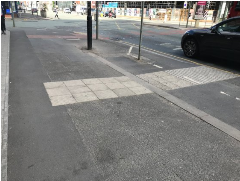
Figure 5: Corduroy surface used in place of ladder surface and not extending across the full width of the footway.
