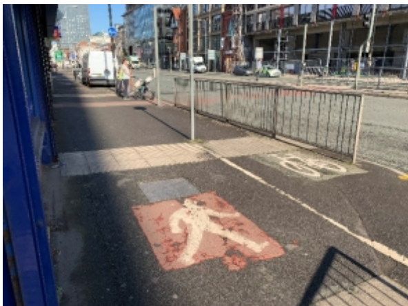
Badly specified parallel footway/cycleway: corduroy used in place of ladder and no delineator strip.
