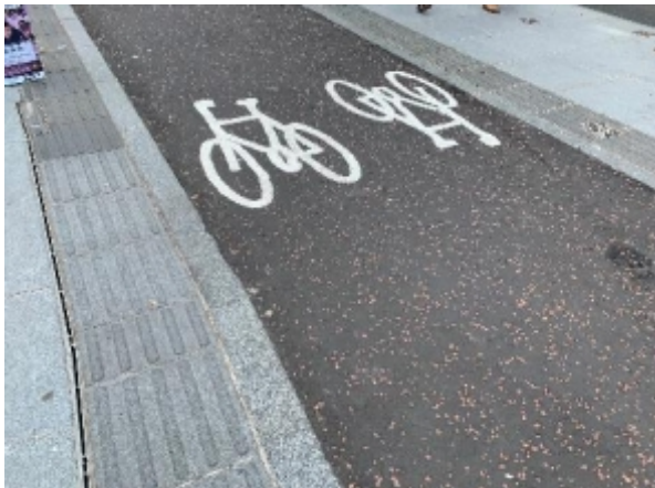
Guidance path surface (400mm depth) used to delineate the edges of a footway level cycle track
