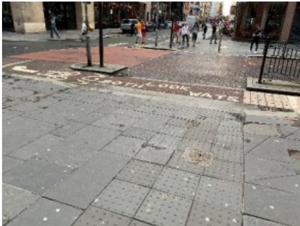
Non-contrasting blisters used for both edge and stem at a signalised crossing
