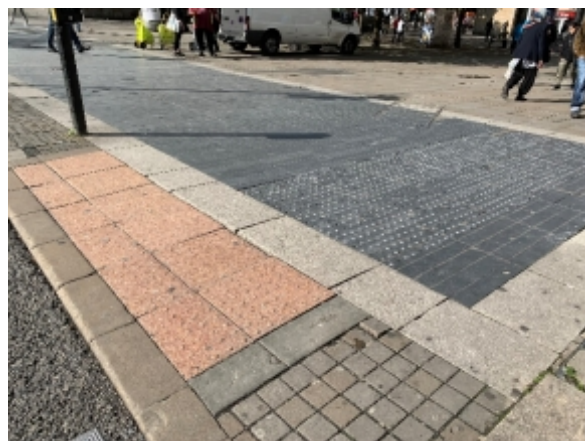
Badly worn blisters at controlled crossing with stem formed from metal studs, many of which are missing
