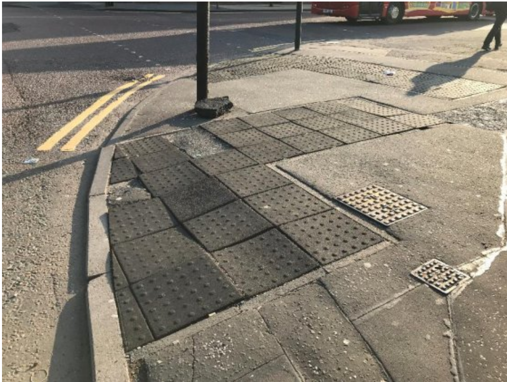
Figure 1: Experimental rubber-based blister paving still in situ, despite failing.
