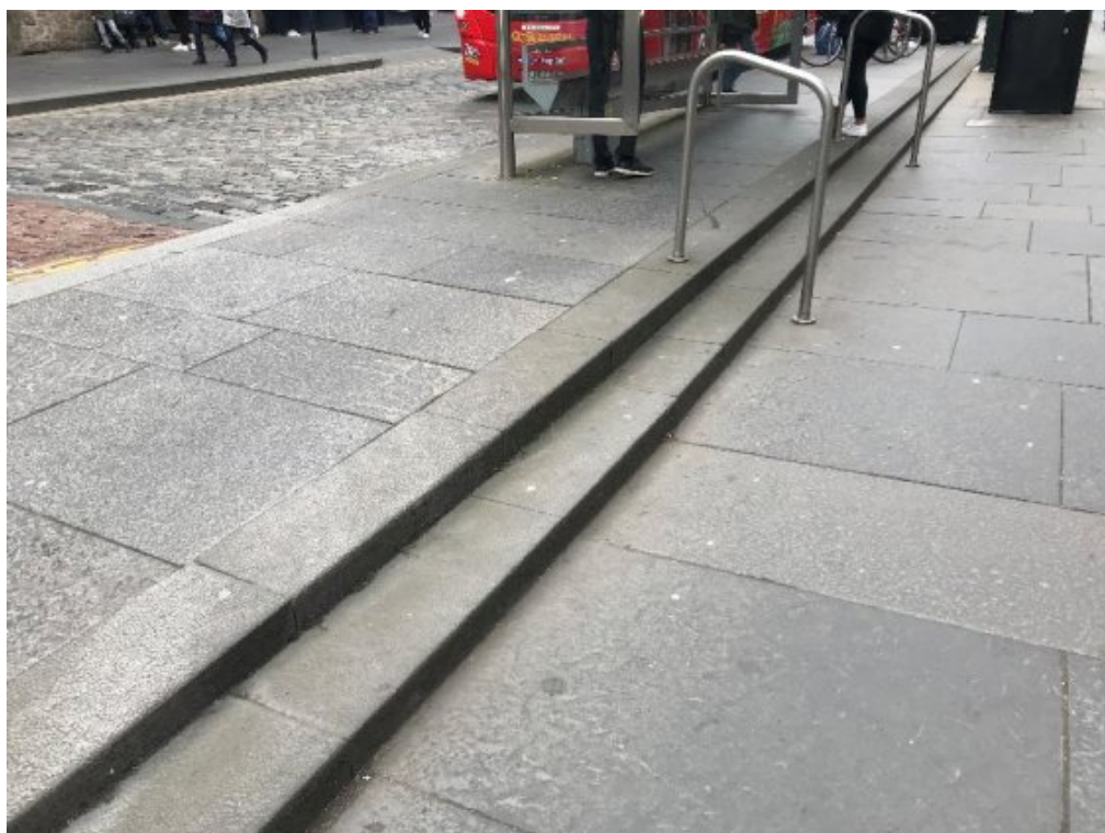
Figure 6: No tactile (corduroy) marking of steps at bus stop. Heritage area.
