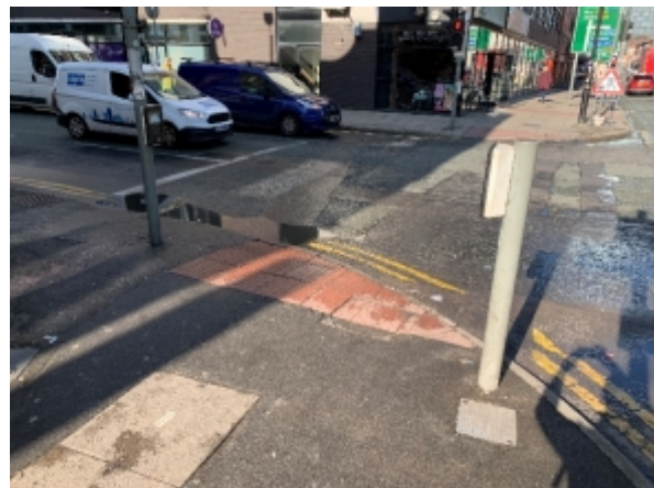
Blisters at signalised crossing with no stem and significant section well below 800mm in depth.
