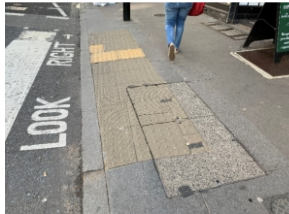
Poorly-contrasting stick-down tactiles at a zebra: helps cover utility trays, but no stem.
