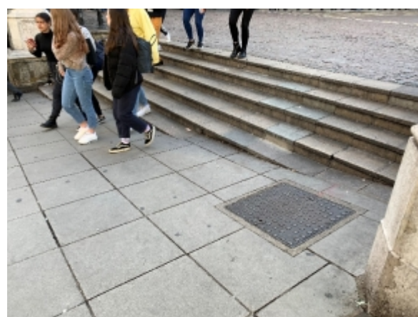
No corduroy provision at top or bottom of these 'fading' steps
