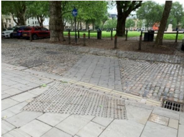
Metal stud blisters on uncontrolled diagonal crossing with starts/lands (near side) in cycling path
