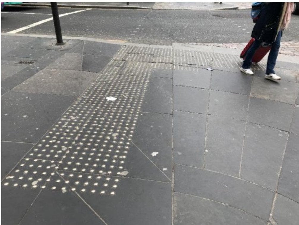
Figure 4: Blister surface formed of metal studs set into stone slabs. One-off public realm scheme in heritage area.
