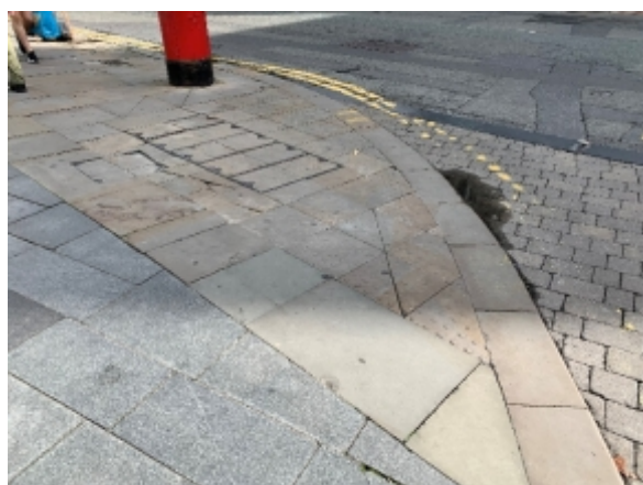
Confusing, poorly-contrasting, worn blisters, with insufficient coverage for both crossing directions
