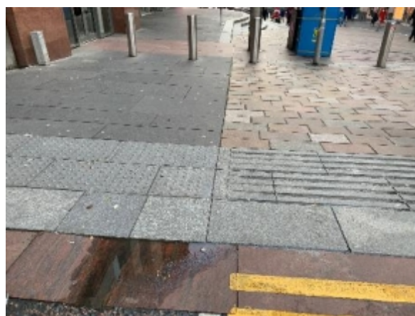
Blister paving at a signalised junction alongside non-standard ribbed paving over nominal vehicle path
